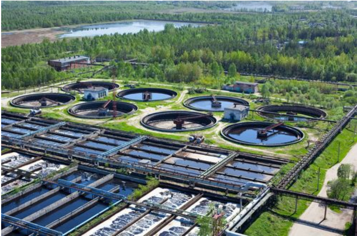
Figure 8: Aeration tanks at water treatment facility (i.e., mechanical, biological, and sludge treatments)
