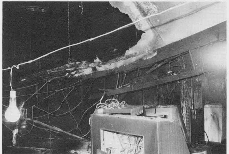
The south side of the planetarium shows clearly how extensive the damage was.
