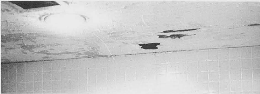
"This building is literally decaying around us."—Tony Sartori
