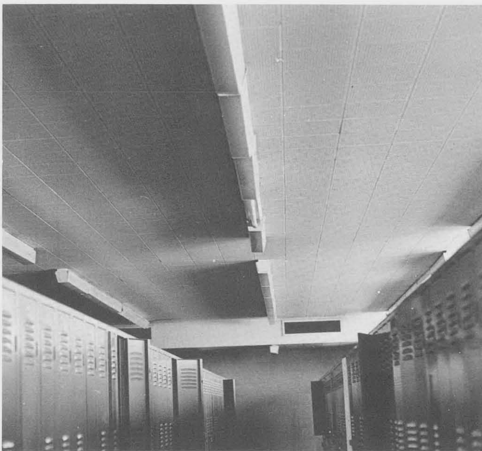
Lights that won't light are just one of the many problems plaguing the existing gym facility.
