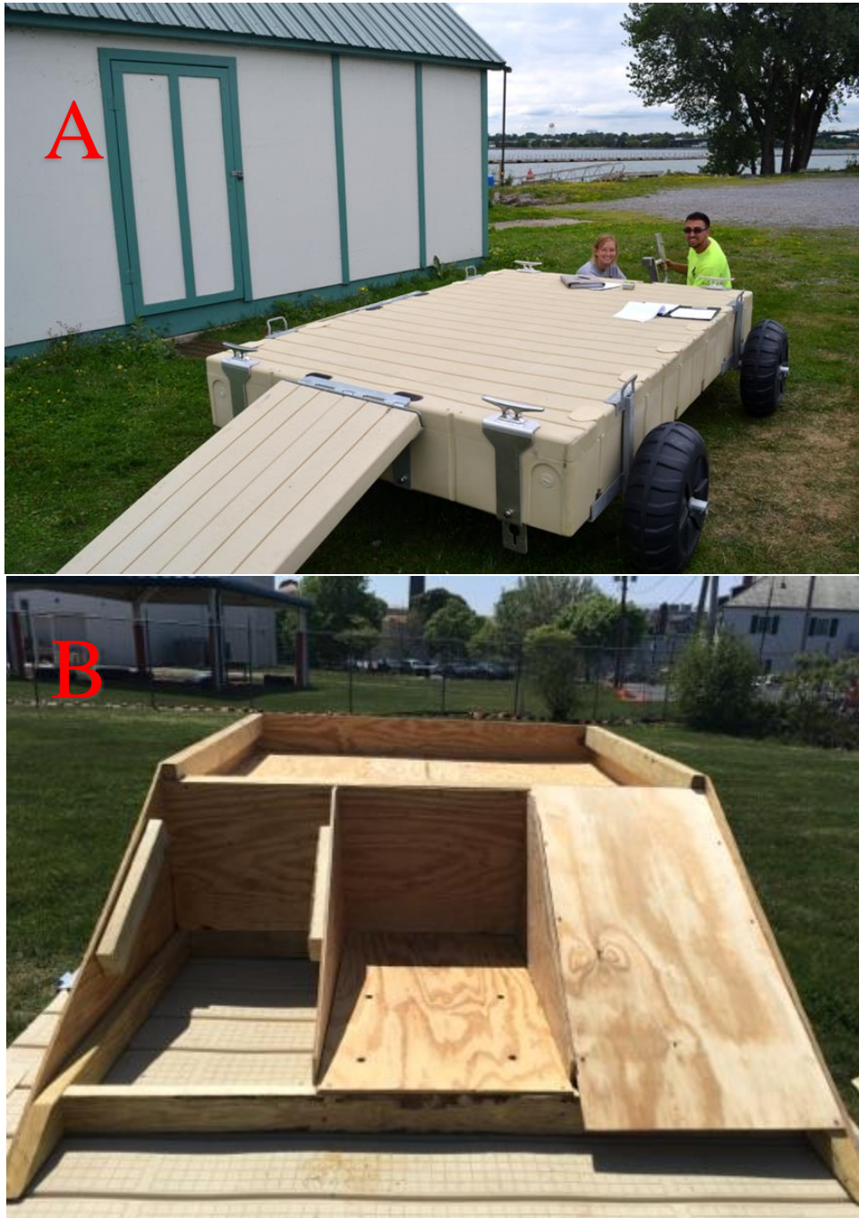
Figure 5. Construction of the basking/nesting platforms. A) Initial construction of platforms. EZ dock base with ramps and wheels. B) Near complete nesting box structure, hard ramps on either side of the center compartment for a sand ramp.
