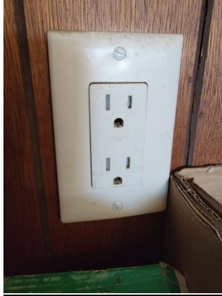
Figure 8: NEMA 5-15 wall outlet. (Own photo, 2021)
