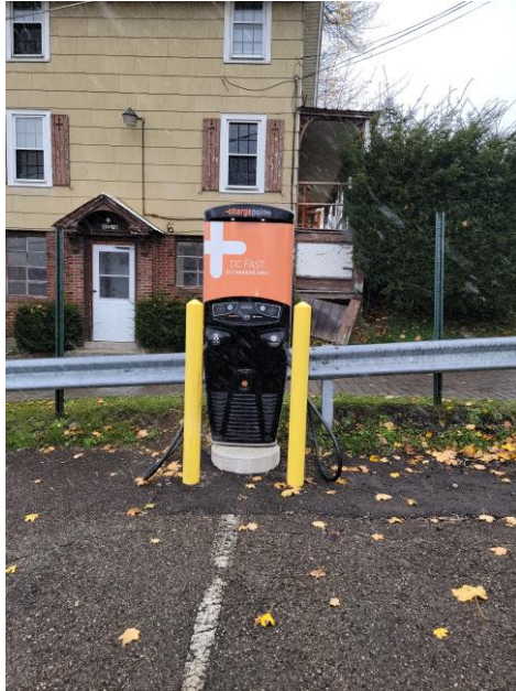
Figure 16: Chargepoint Network (DC Fast Charger). (Own photo, 2021)
