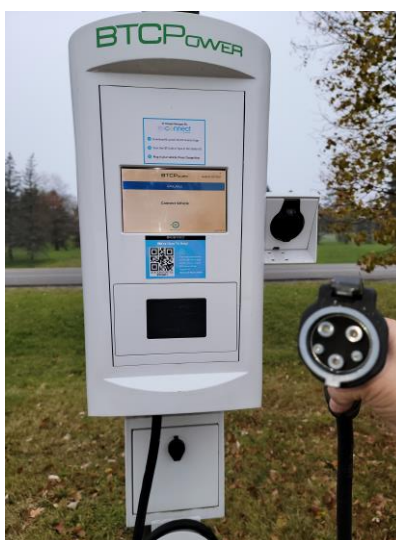
Figure 19: BTCPower powered by EV Connect (Close-up w/ J1772 Plug). (Own photo, 2021)
