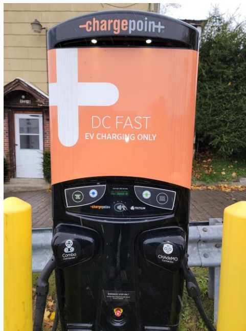
Figure 17: Chargepoint Network (Up-close With both DC Combo and CHAdEMO plug). (Own photo, 2021)
